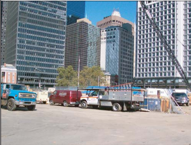
Whitehall Ferry Terminal construction staging area in Peter Minuit Plaza, looking northeast.
