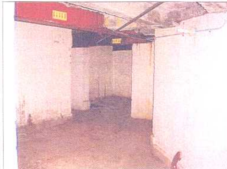
PHOTO 6- INSIDE VAULT, CORNER OF GREENWICH STREET AND BATTERY PLACE FACING NORTHWEST AT STAIRWELL
