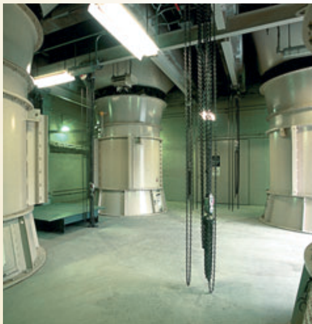
Fan plants are part of the invisible infrastructure improved by the Capital Program.
