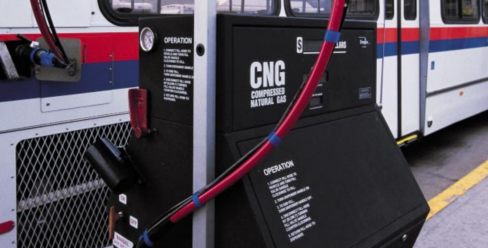
CNG refueling at the natural gas bus depot in Rockville Centre
