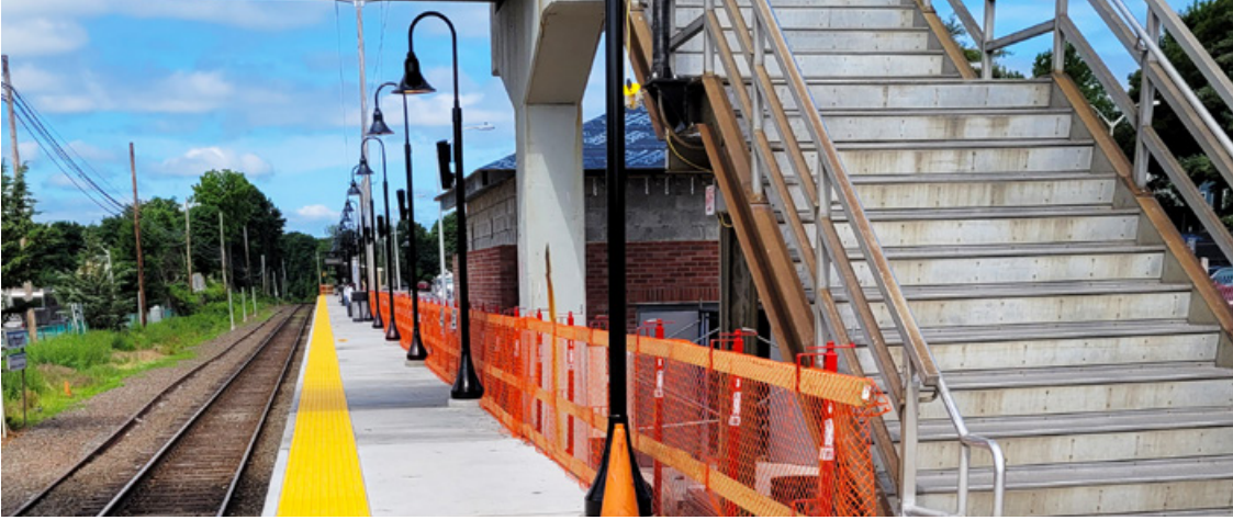
Phase 1 of platform work at Northport Station is now complete and Phase 2 is underway.
