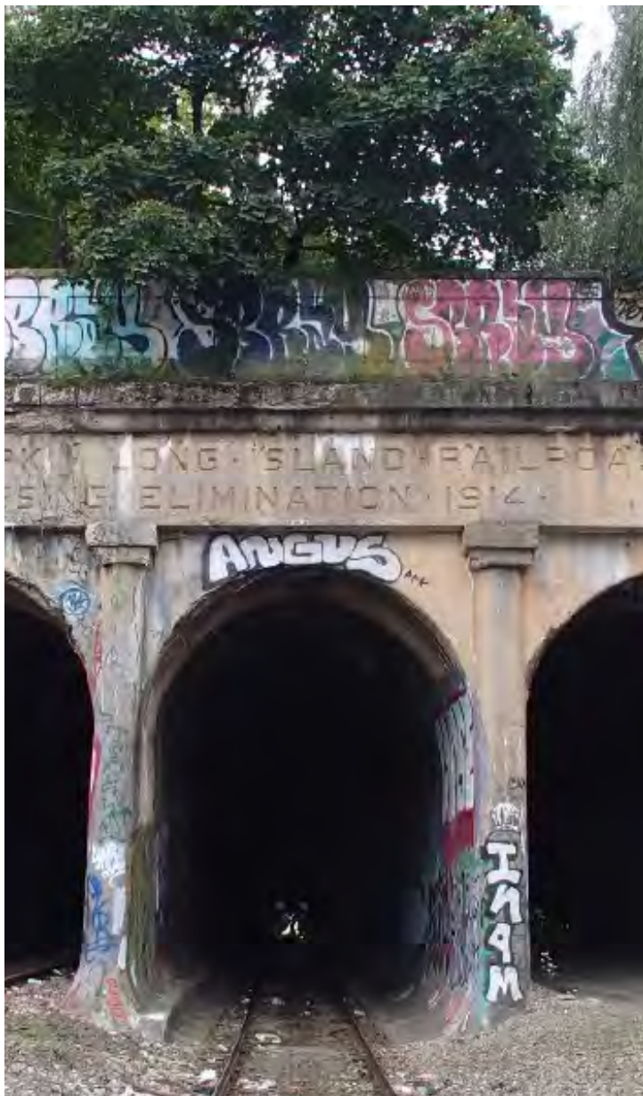
The East New York Tunnel, constructed over 100 years ago, would be rehabilitated for IBX service.
