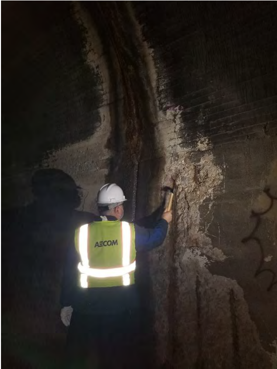
Picture 8 – Spalling and rebar deterioration at a concrete joint
