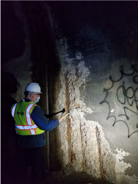
Picture 7 – Western tunnel looking at concrete spalling and deteriorated rebar
