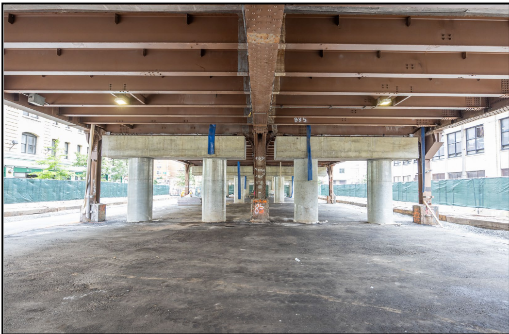
Finished Lot Beneath the Viaduct Between East 130th Street and East 131st Street
