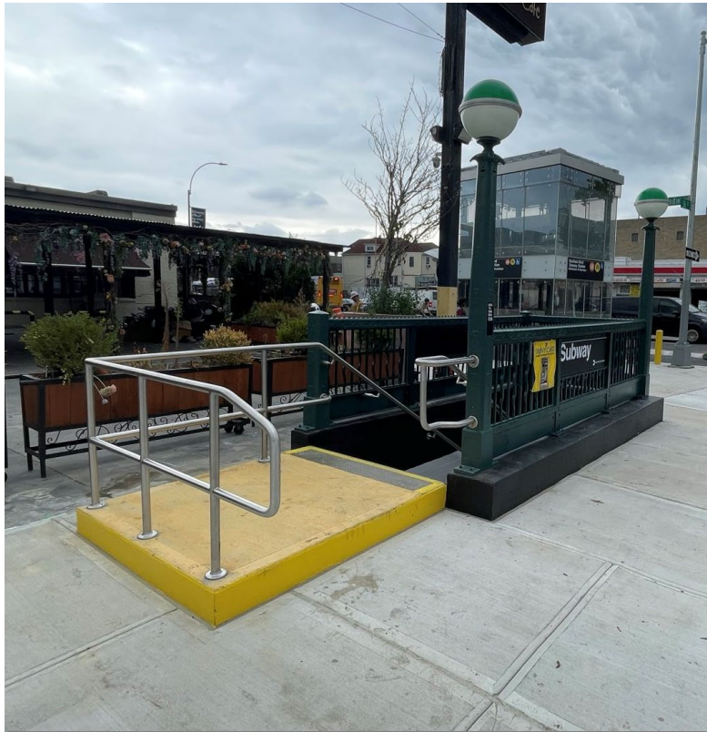
1. Keep stormwater out Install stormwater runoff protections like new top step at Northern Blvd M R
