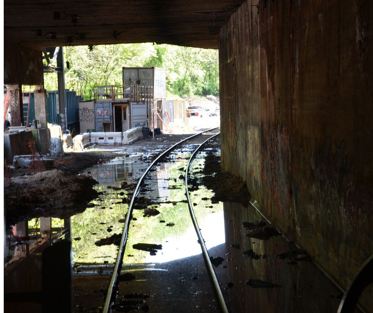
Track Ponding at Entrance to 65th Street Yard
