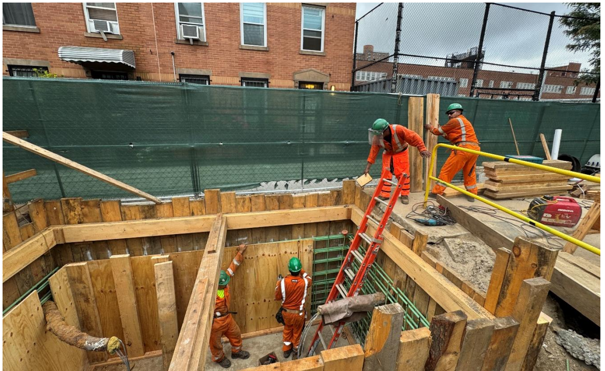
Workers build a new Electrical Utility Vault on 110 th Street between 2 nd and 3 rd Avenue
