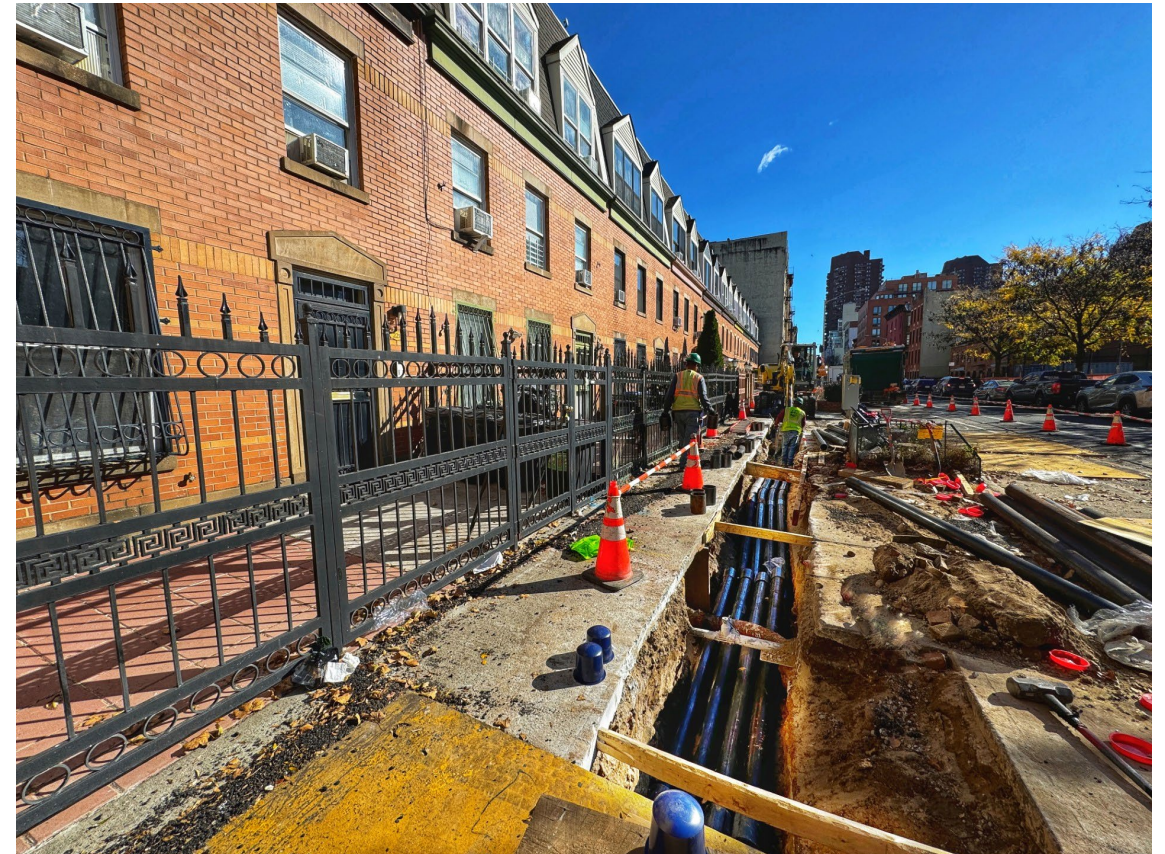
110 th Street between Second and Third Avenue- Electrical duct
