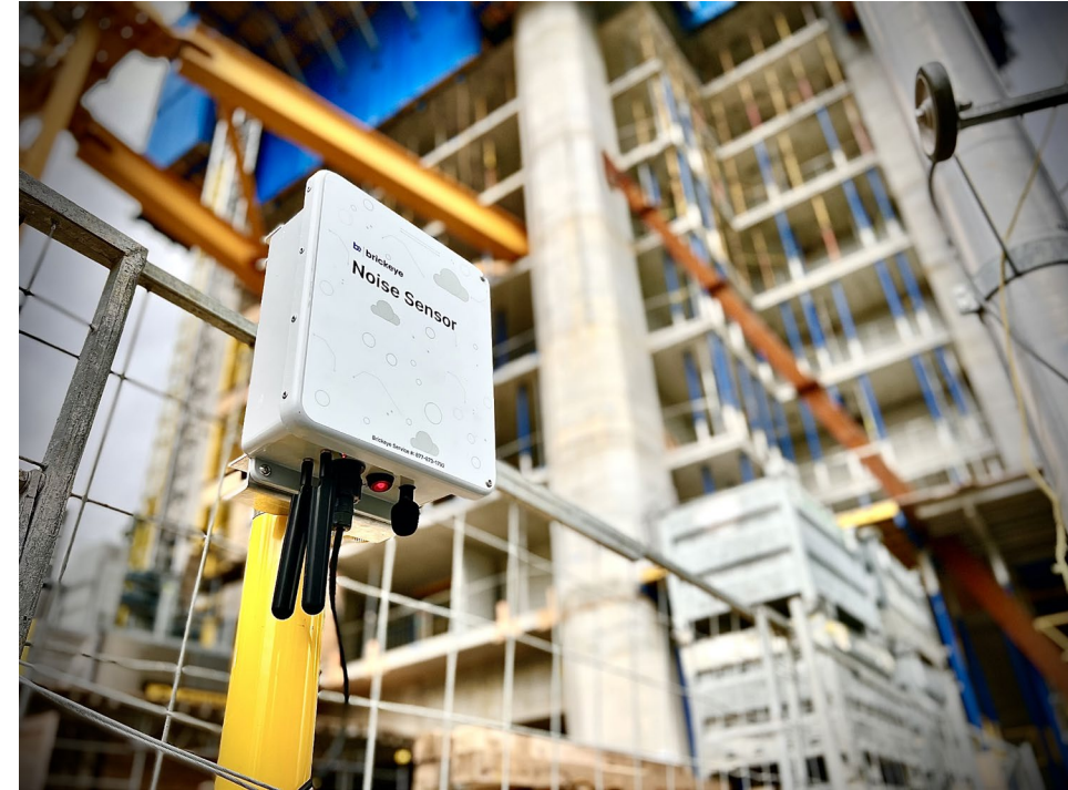
Noise Monitoring Device
