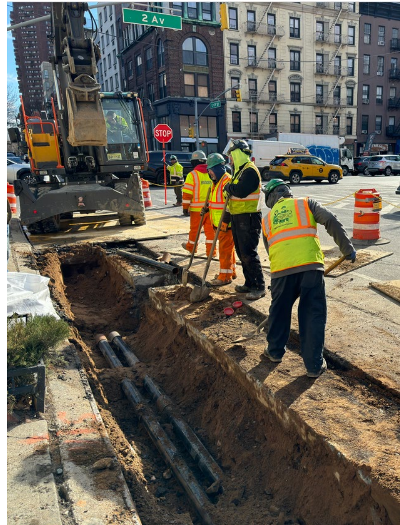
109th Street - 1st & 2nd Avenue- Electrical Duct
