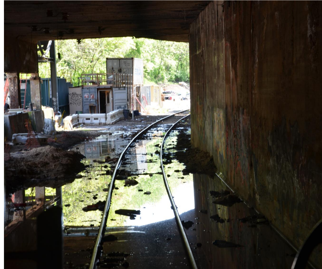
Track Ponding at Entrance to 65th Street Yard
