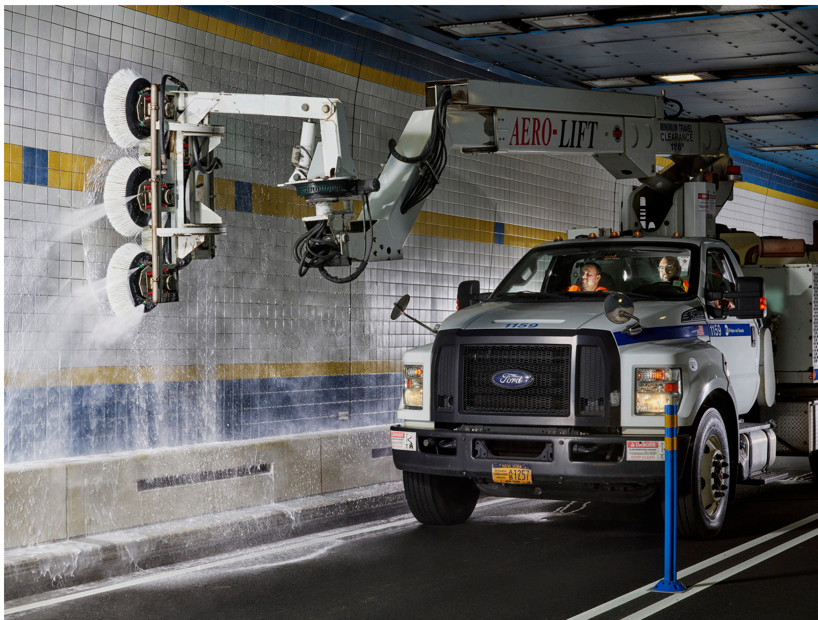
Photograph from the exhibition In Service: MTA Photographs by Christopher Payne, commissioned by MTA Arts & Design.
